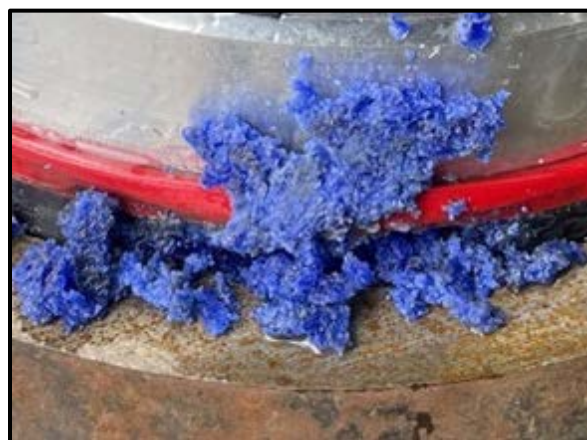
Figure 39: Crumbling of Tri-Ply Seal
