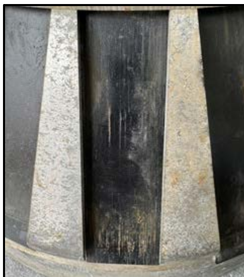
Figure 36: Worn Out And Dirty Back Plate
