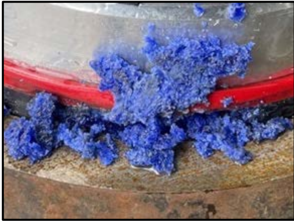
Figure 39: Crumbling of Tri-Ply Seal
