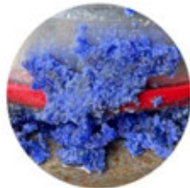
Figure 11: Crumbling of Tri-Ply Seal
