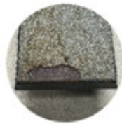
Figure 4: Flaking of GritLock
