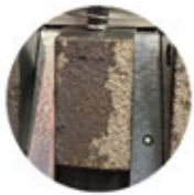
Figure 1: Clogged GritLock Surface
